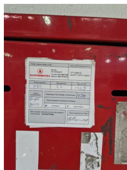
Regularly checked fire hydrant.jpg
